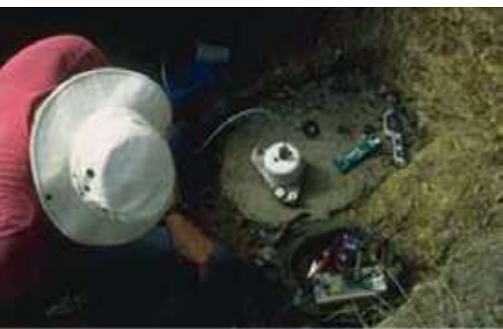
Model 701 Tiltmeter being installed at Soufriere Hills Volcano, Montserrat (Courtesy of USGS)
