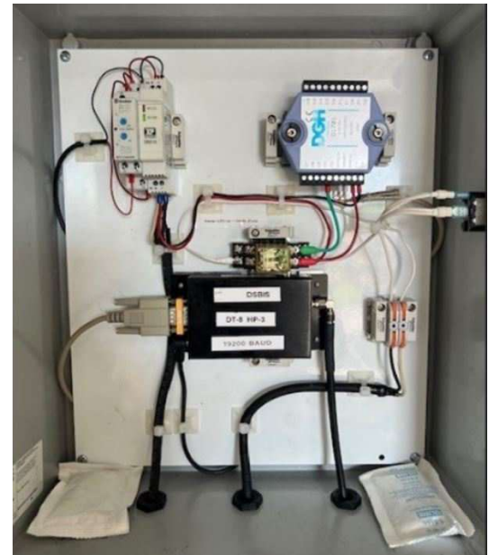
Real-time GPS monitoring system using DGH I/O Modules
