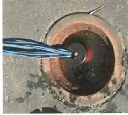
15. Installation complete - string hung from casing hanger and cables fed through opening
