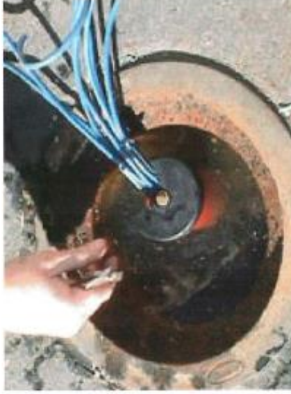
18. Installation complete - string hung from casing hanger and cables fed through opening
